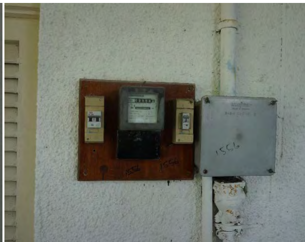
Figure 23: Existing three phase power board at MET Office
