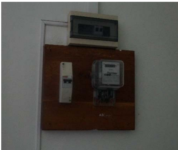
Figure 22: Existing single-phase power board at MET Office Accommodation Block
