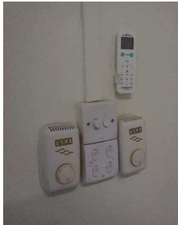
Figure 25: Figure above shows the fan, air conditioning and lighting controls for the office building
