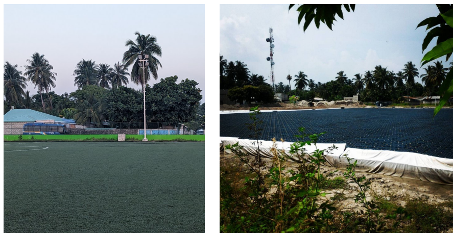
Figure 8: Current ZigZag stadium under which aqua cells are located (left), and aqua cells during construction phase (right)
